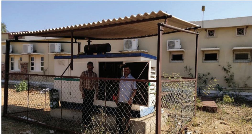
DG set for the centre
