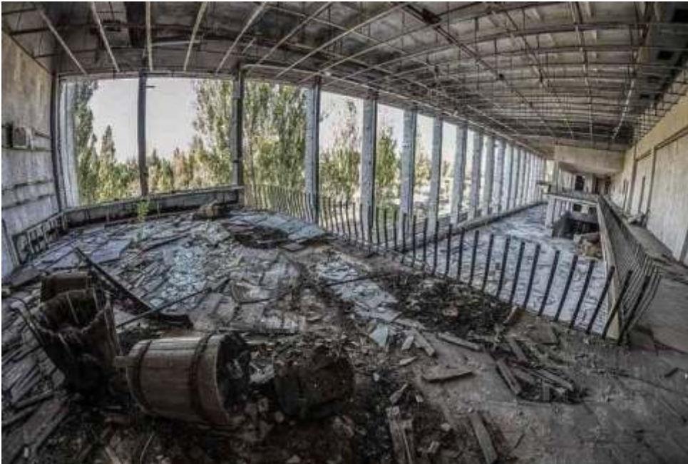
The after damage caused in the factory. Source: defenceworld.net
